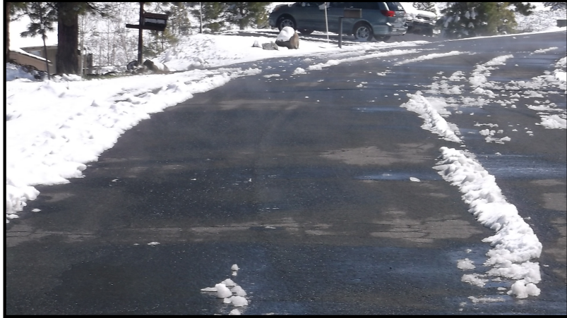
Asphalt on Lance Drive
