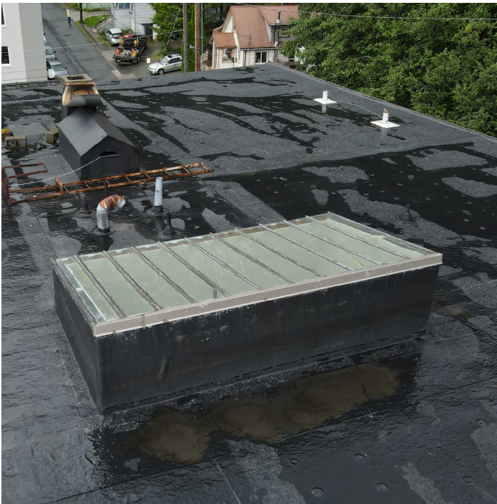
No cricket in front of skylight. Minor ponding concern.
