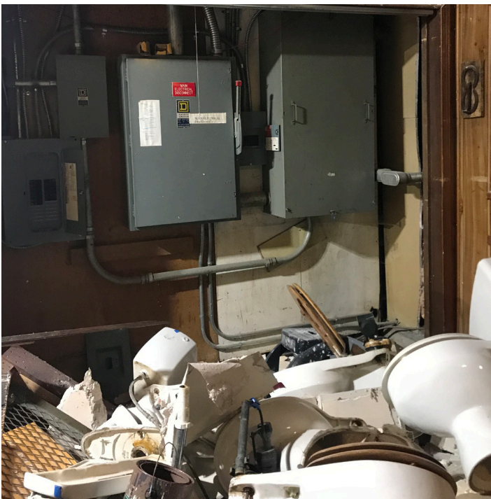
Main electrical shutoff and power in. Appears contemporary and in good condition. We did not ascend toilet mountain to inspect closer.
