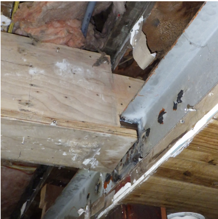
Steel beam and connecting beam above bar on lower level. Beam size and connection unknown and in locations with significant settling. Structural analysis is needed. (paint was not tested for lead.)
