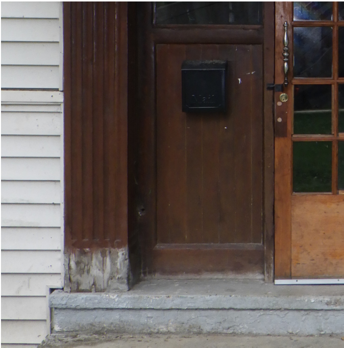
Main south entry detail image. Some water damage at grade that needs repair. Door does not appear original, however, is made similar to historic.
