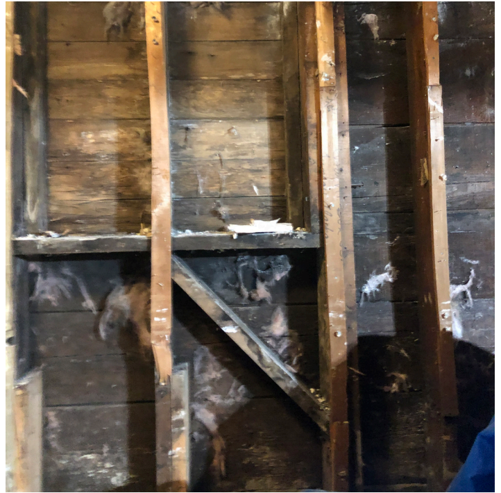
In general, lower level walls have moisture and mold issues that need remediation.
