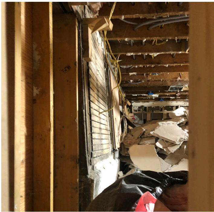
Inside view of landslide damage. If shored properly, this may be of historic merit for renovation.
