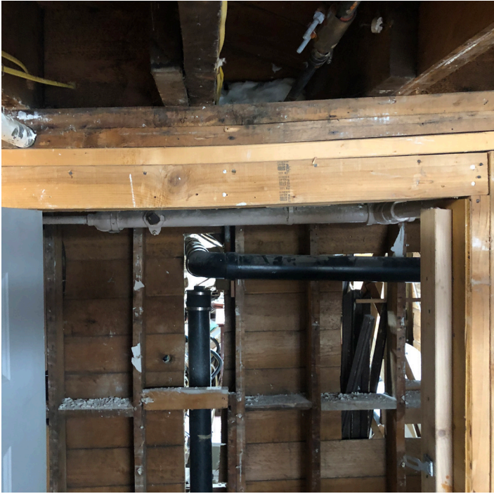
Sagging header above door to workroom. Telltale sign this is a bearing wall.
