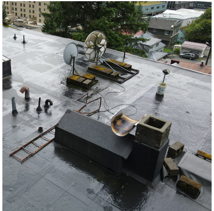
No crickets. Chimney cap blown off. Recommend replacing chimney cap.
