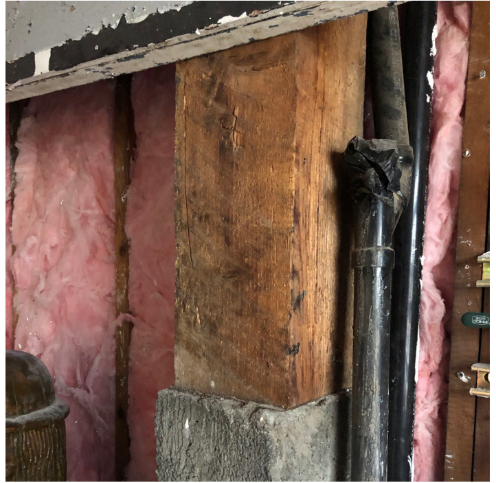
Many of the older historic timber columns only have gravity connections. Not to current seismic code.
