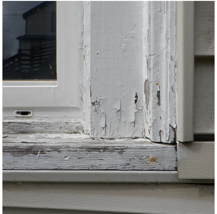
Window detailing. Contemporary vinyl window with painted wood trim surround. Wood trims appear to be historic in style, though no exact record of detailing was found.
