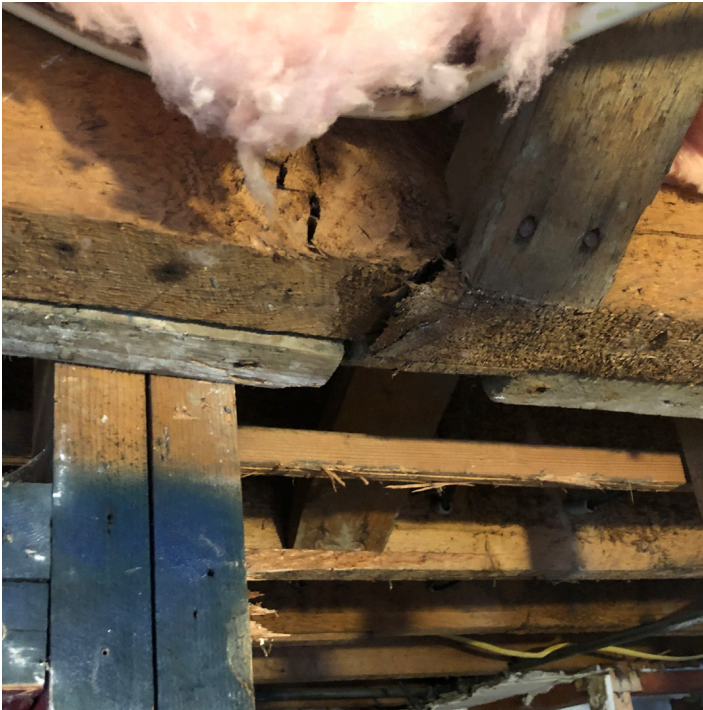
Load bearing joist/beam failure near work room. See drawings for callout.
