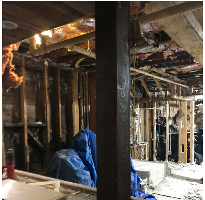
Timber column appears to be taking load of major steel beams at lower level bar. Structural analysis needed.
