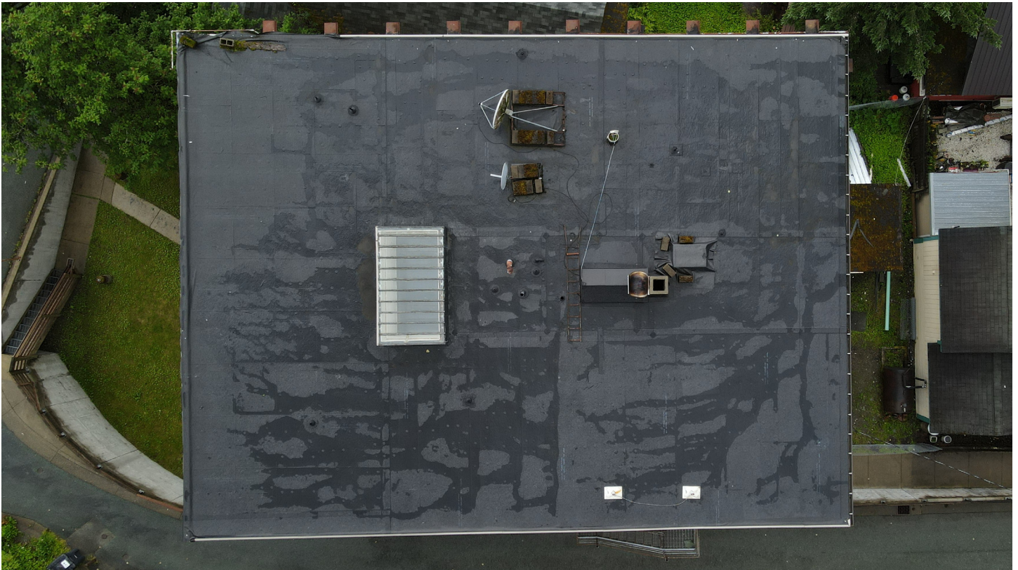
Roof drone photo. Drainage pattern make settling of building apparent. Roof membrane appeared in good condition. Penetrations appeared fully wrapped or termination bars are in place and functioning.
