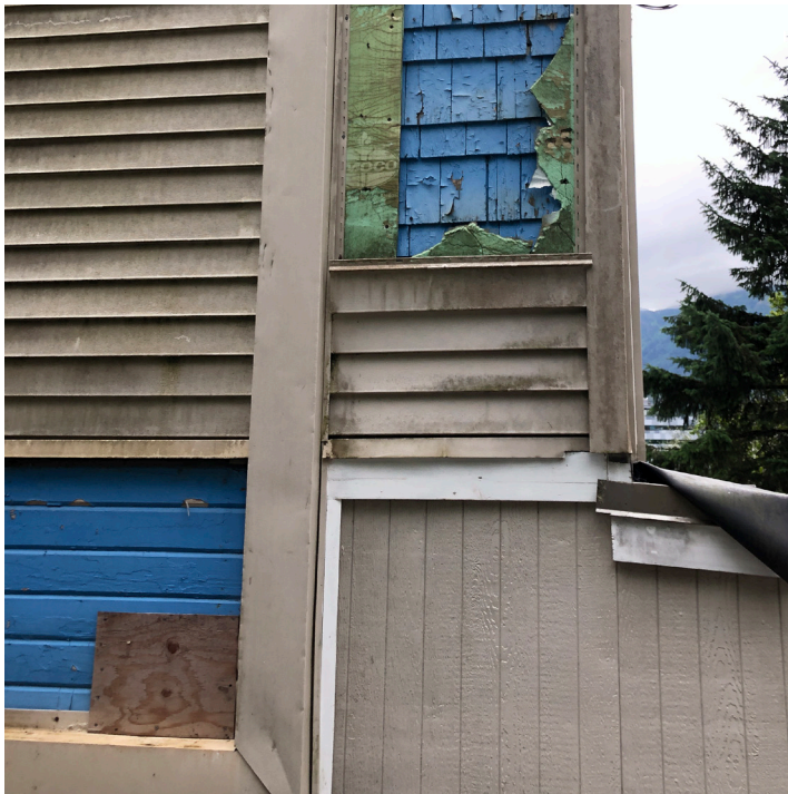
Differing vintages of siding, and added exterior items such as conduit flashing for lighting. Recommend full tear off and new exterior envelope.
