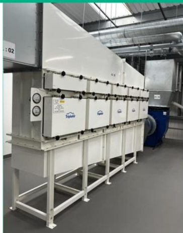
HEPA Bank for extracted air
