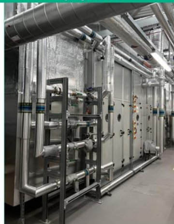
Air conditioning for incoming air, including Humidity, purity and flow
