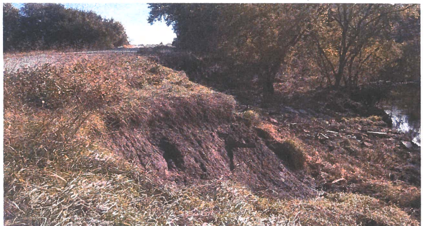
Brown County EWP exigency streambank stabilization. High traffic county roadway impacted by flooding.
