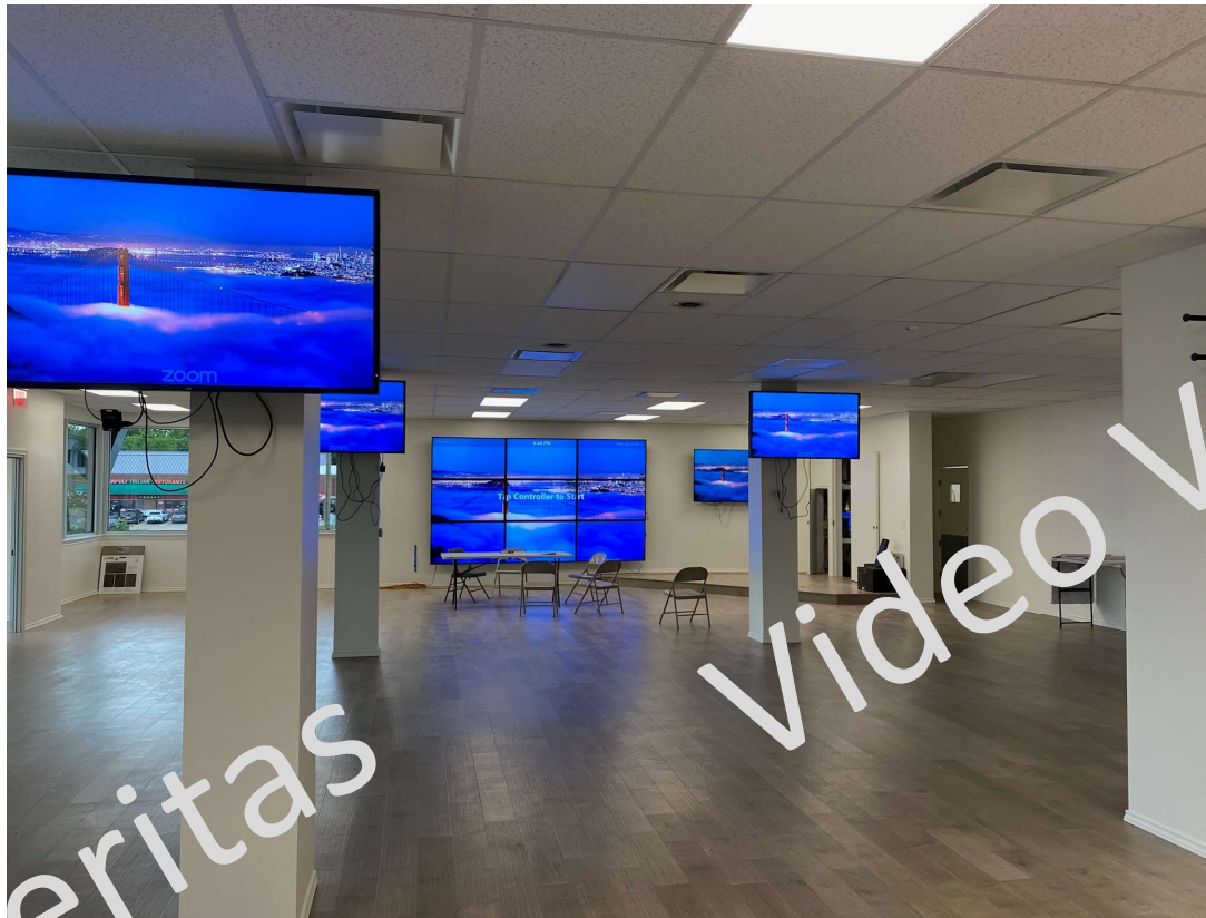
As-Built Diagrams for Audio Visual System Rockwall Noon Rotary, Rotary Hall 408 S. Goliad, Rockwall, Tx
