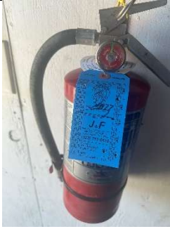
Fire extinguisher expired tag
