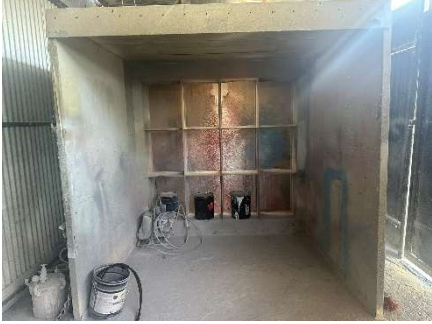
No Automatic Extinguisher System in Spray booth
