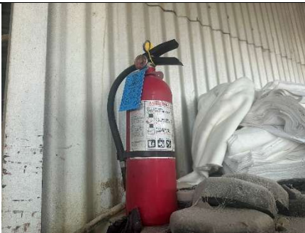
Fire extinguisher not mounted
