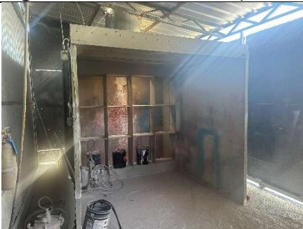
Missing filters in spray booth
