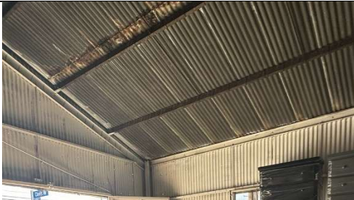
Roof Rust / Corrosion
