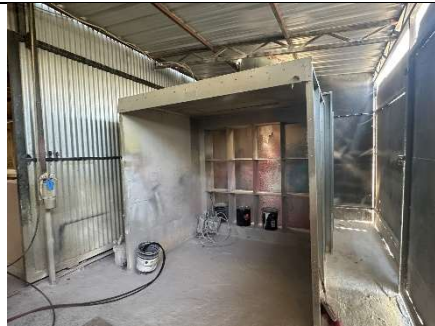
Missing filters in spray booth
