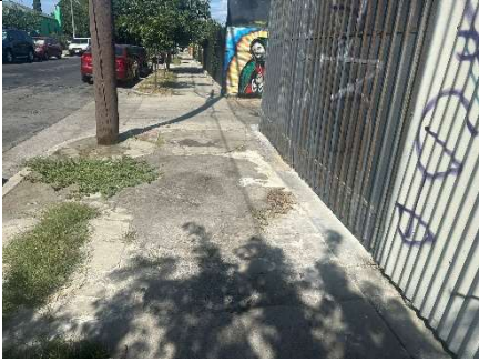
Cracked sidewalk on left side
