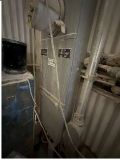
Obstructed electric panel
