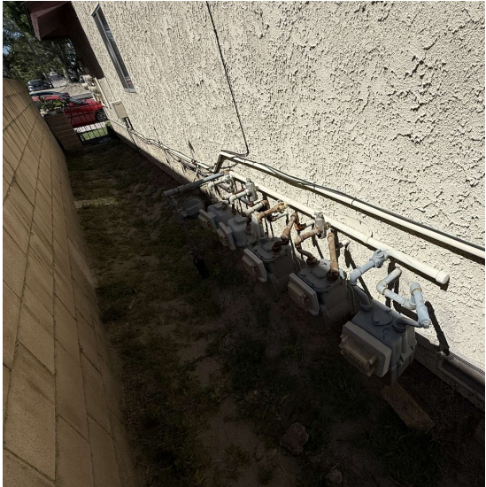
Gas meter with no earthquake shut off valve
