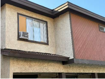
No bracing for window AC unit
