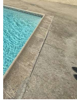
Missing depth markers
