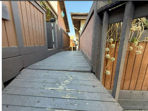
Uplifted section of wood deck
