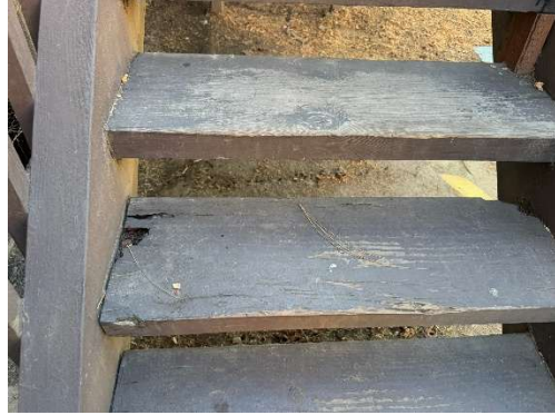
Cracks in steps
