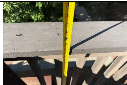
Balcony railing height 34" tall
