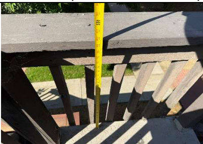
Balcony railing height 34" tall
