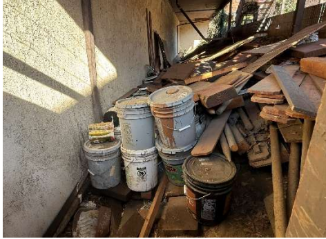
Stored debris near unit 27
