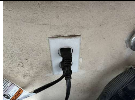
No GFCI Installed near washing machine
