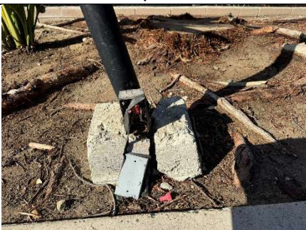
Exposed junction box
