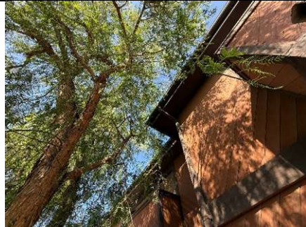
Tree overhanging building
