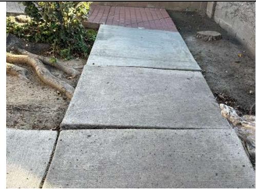
Uplifted section of concrete walkway
