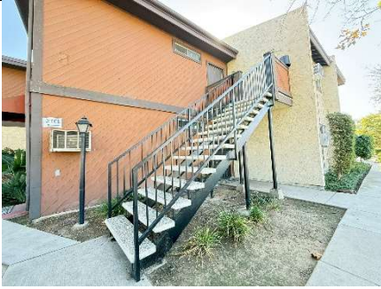
Missing fire extinguishers on 2 nd floor
