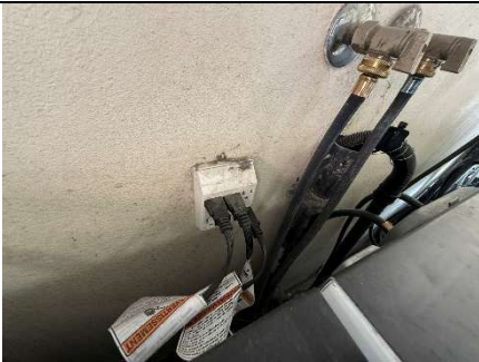
No GFCI installed near washing machine
