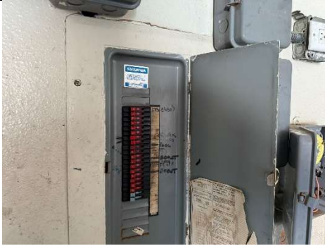
Circuit breaker panel
