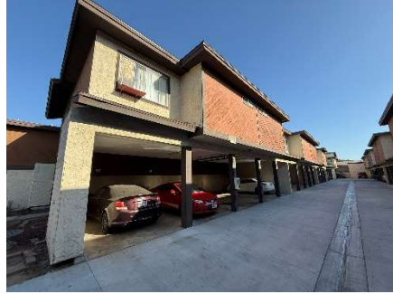
No bracing for window AC unit
