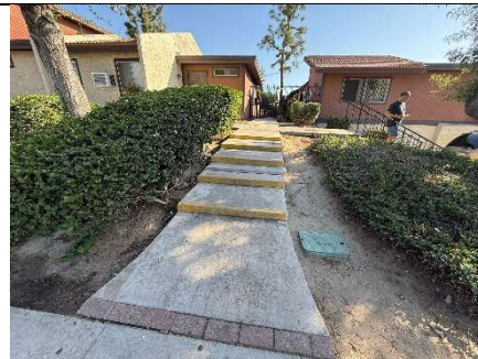
Missing rails on steps
