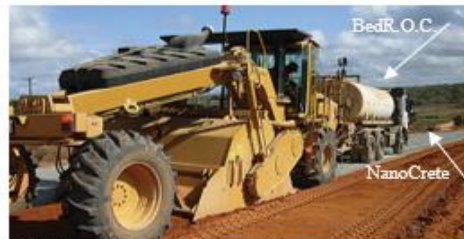
5. In Situ mix into soil with reclaimer or equivalent. Pro-SealECCO NanoCrete & Pro-SealECCO Bed-R.O.C. the Pro-SealECCO Secondary Containment barrier.
