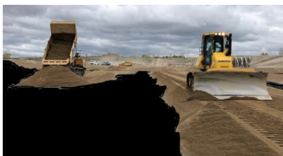
12. Cover and place recovery systems in and over cover soils and rock
