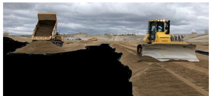
Cover Pro-SealECCO leachate collection system, applied over Pro-SealECCO stabilization with protective soil layer.
