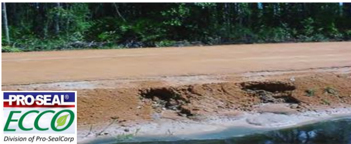
(Above) this road base is placed in extreme wet environs. Table (below) displays the results of Atterberg Limit and Plasticity testing for natural wet soils mixed with the Pro-Seal ECCO® Stabilization System containing >16% minimum +4%
