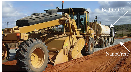
5. In Situ reclaim into soil Pro-SealECCO NanoCrete® & Pro-SealECCO BedR.O.C. the Pro-SealECCO Secondary Containment barrier
