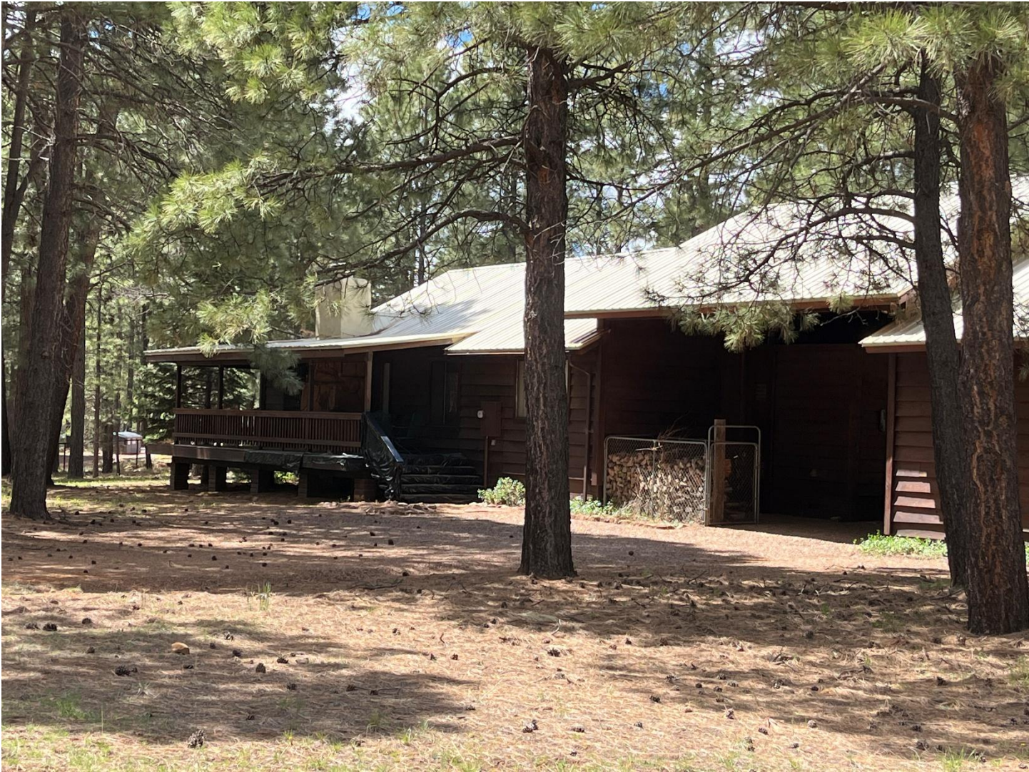
Firewood pile up against structure with needle layer around it.
