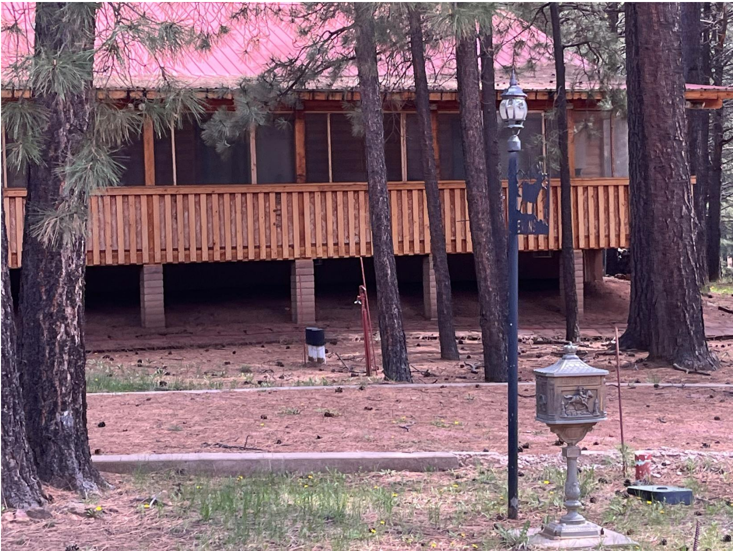
Deck height is good compared to needle cast. Minimal to no combustible material underneath the deck.
