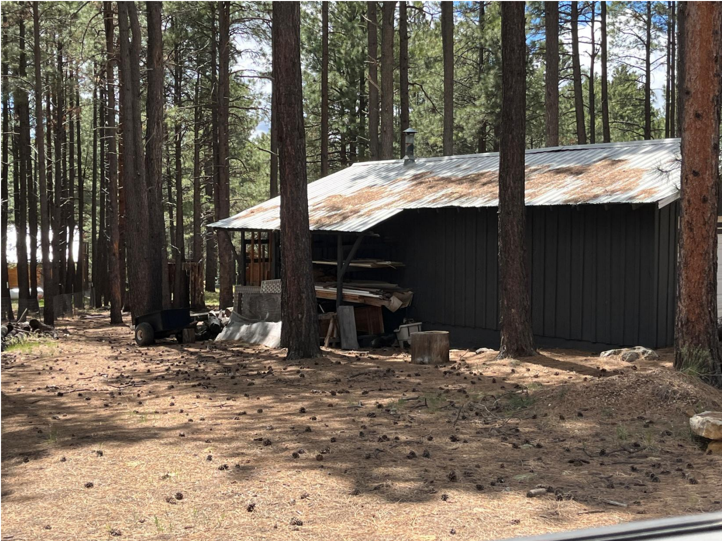
Photo includes needle layer on metal roof and combustible material up against the wall. There also is a thick needle layer leading up the siding of the structure.
