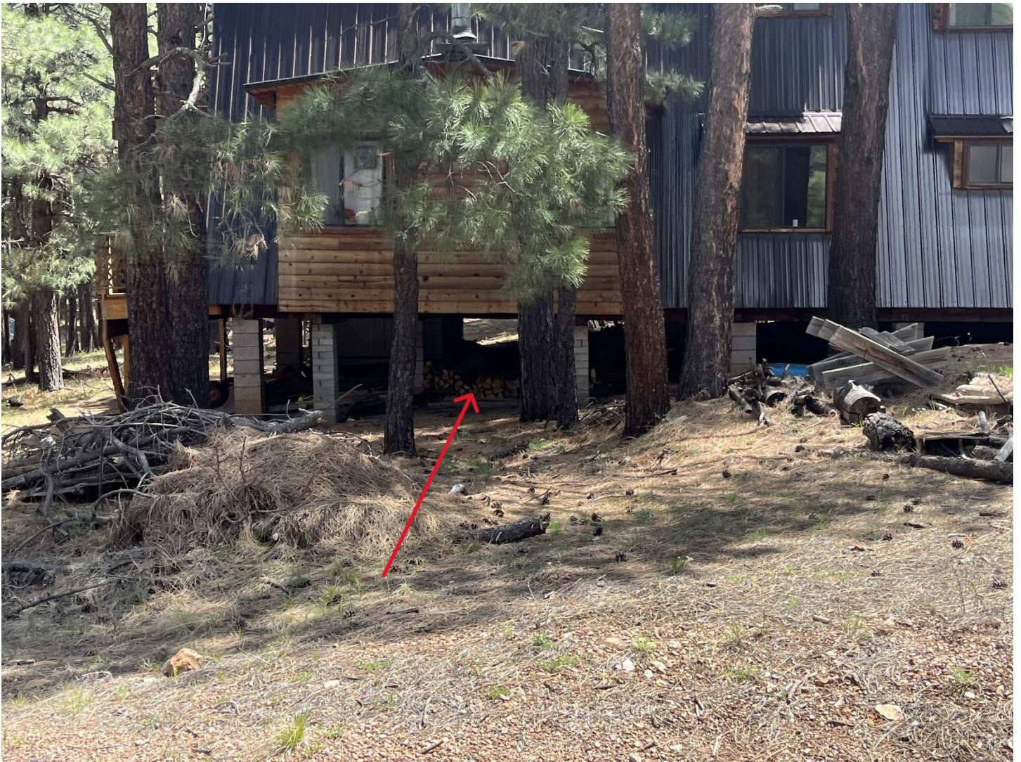
RED arrow identifies a firewood pile underneath the main home. This is a receptive fuel bed for fire embers to land and ignite.
