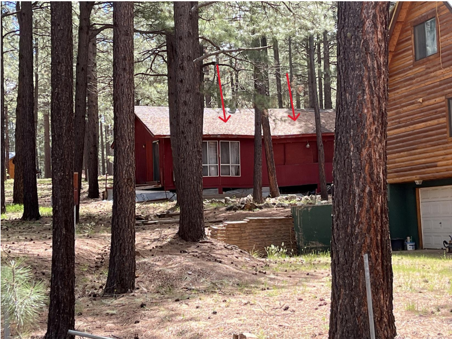
RED arrows identify needle layer on asphalt single roof.
