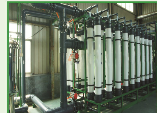
Ultra Filtration System
