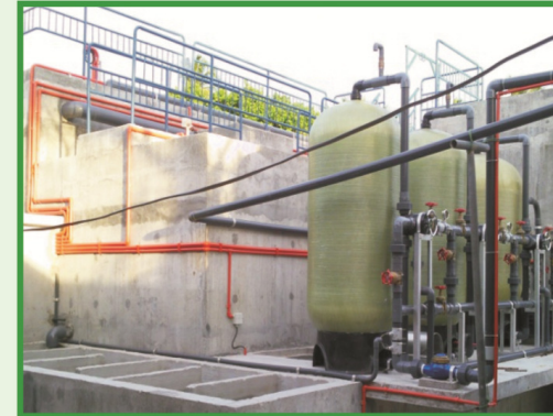
Civil ETP / STP Plant
