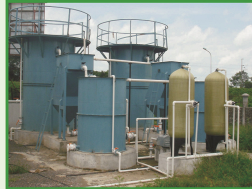
Fabricated ETP / STP Plant
