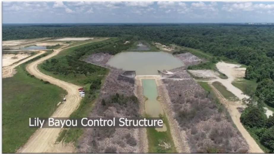
Screen capture from the USACE's Project Update Drone Flight from July 2023 showing progress near the Lily Bayou Control Structure.
