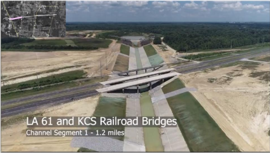
Screen capture from the USACE's Project Update Drone Flight from July 2023 showing progress near LA 61 and KCS Railroad Bridges.
