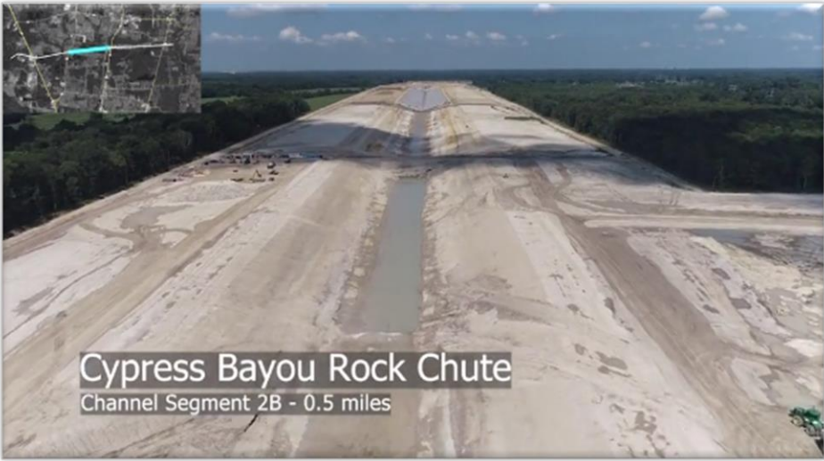
Screen capture from the USACE's Project Update Drone Flight from July 2023 showing progress near the Cypress Bayou Rock Chute.
