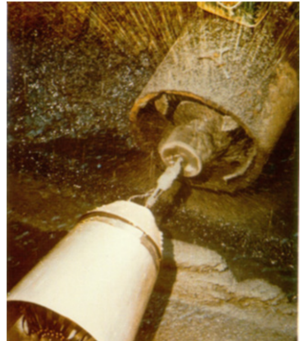
A thin layer of cement (1/4 inch) between the water and the metal of the pipe keeps minerals from building up to the point of restricting the flow.
