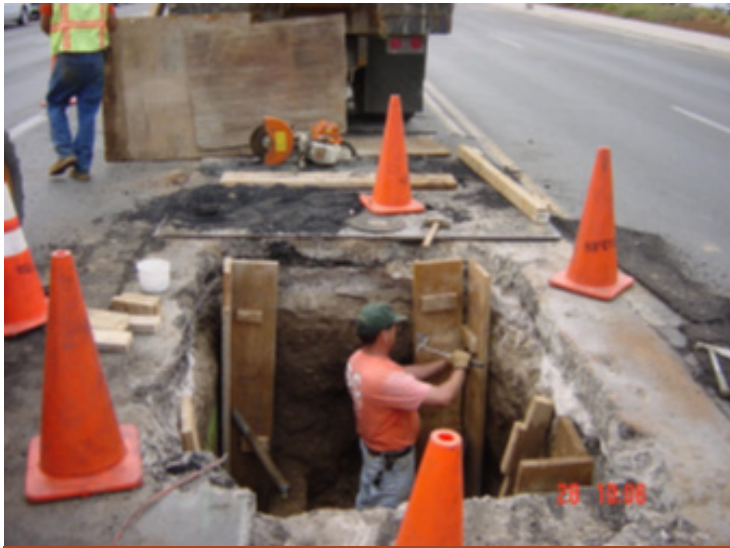
A small excavation is made at each end of the main to be lined. This is what it looks like by day in the street while crews work.
