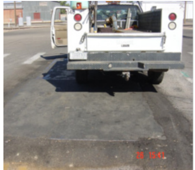
Travel during non-work times is virtually seamless where excavation is covered by a steel plate
