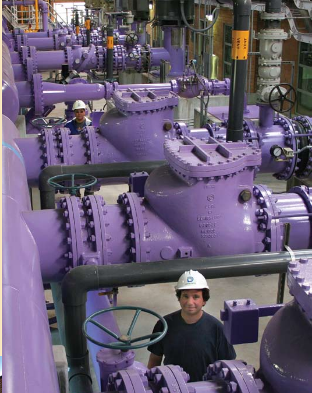
Employees in the Denver Water Recycling Plant stand inside the plant, which was built in 2004. Recycled water pipe is colored purple to help distinguish it from potable water pipe.
