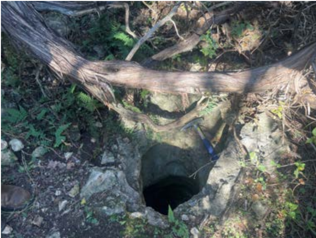
Photo 9 – Location BB-13 – Sinkhole feature. Opening is approximately 0.5 meter by 0.25 meter.
