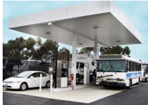
A compressed natural gas (CNG) fueling station at UC San Diego's Energy Innovation Park is used by the campus fleet of CNG delivery trucks, street sweepers, sedans, pick-up trucks and buses. Photo credit Rhett Miller, UC San Diego
