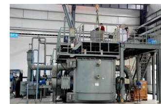
速凝薄带炉 Strip casting furnace
