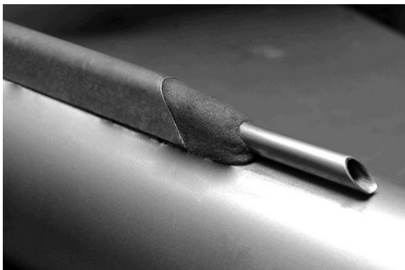
Figure 3: Cured mastic now creates uninterrupted thermal connection between tracer and pipe wall
