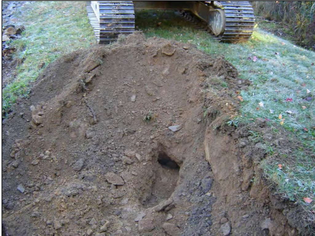
Photo 5: Excavation followed the seepage path. At this point it opened up to nearly the size of a basketball.
