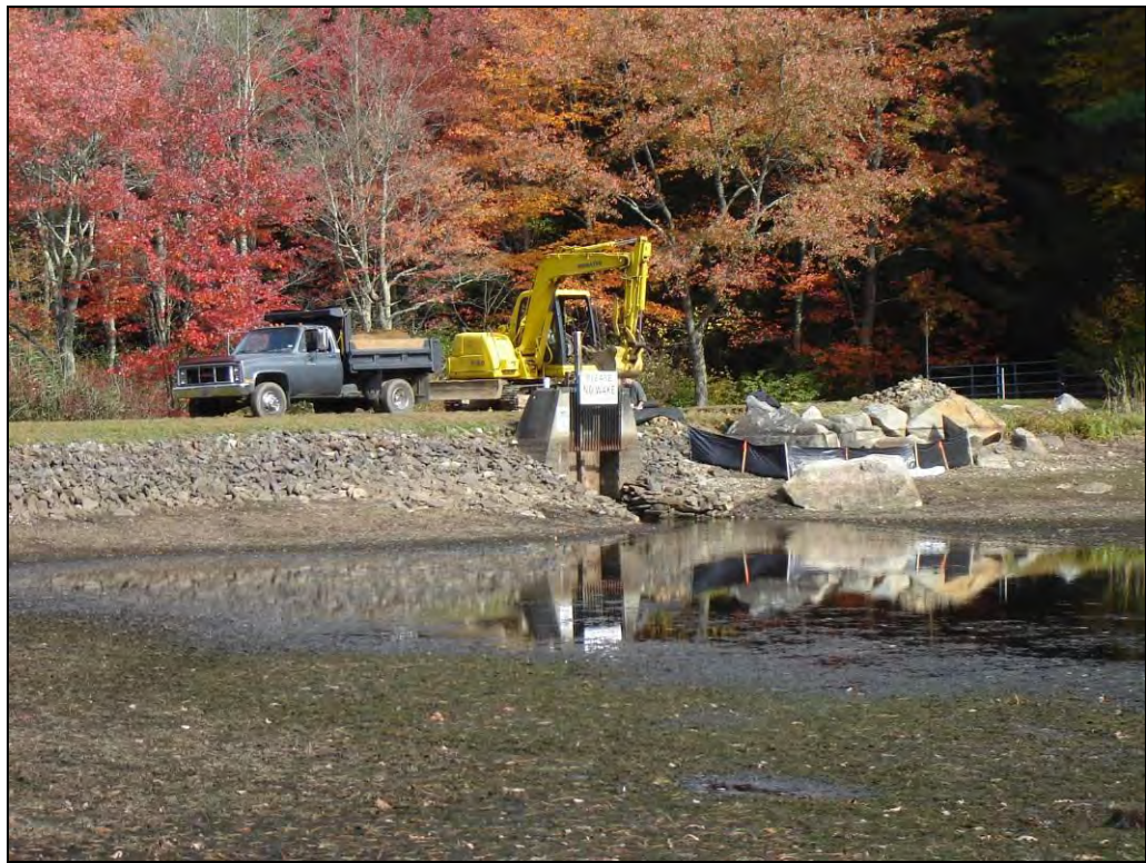
Photo 2: Overview of construction location on dam, right of low-level outlet intake riser.
