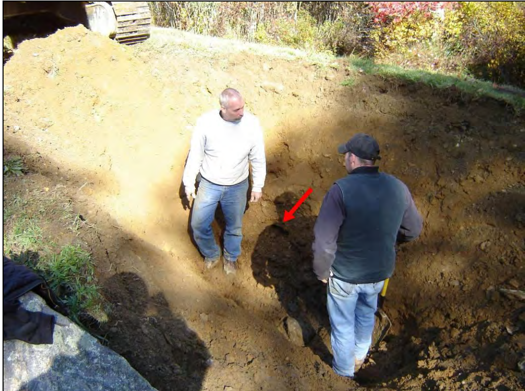
Photo 7: Location of seepage path exit point on downstream face of excavation
