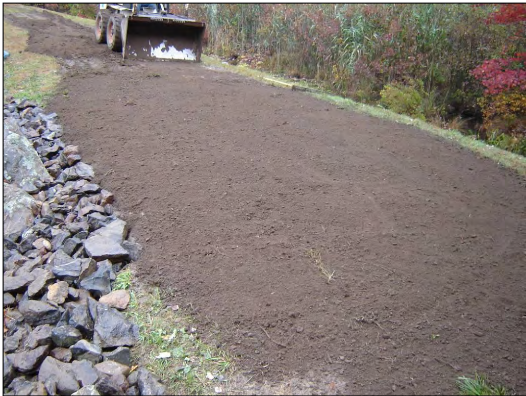
Photo 14: 4-inch layer of topsoil placed and seeded over excavation site and to fill ruts from machinery.
