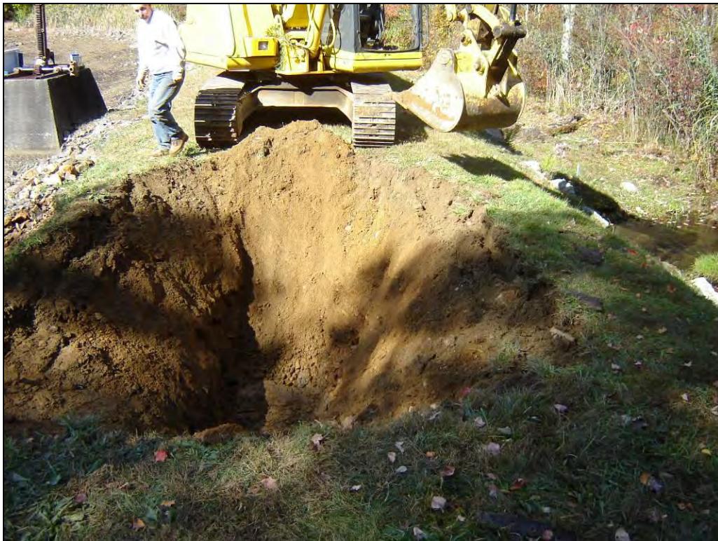
Photo 6: The completed excavation retained intact embankment on the downstream side and along much of the upstream side.
