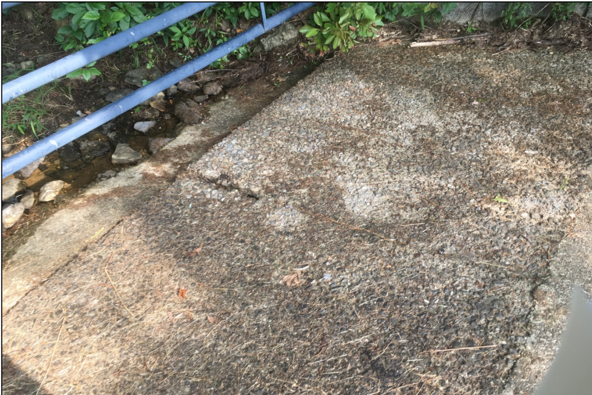
Photo 17: Overview of weir, note the differential settlement on the slab.
