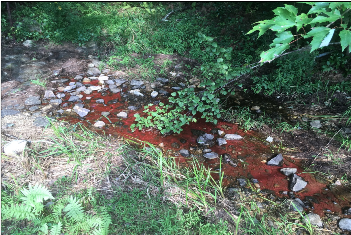
Photo 18: Overview of downstream channel at primary spillway. The water is colored with excess dye that was used to assess leakage at the upstream side of the dam.
