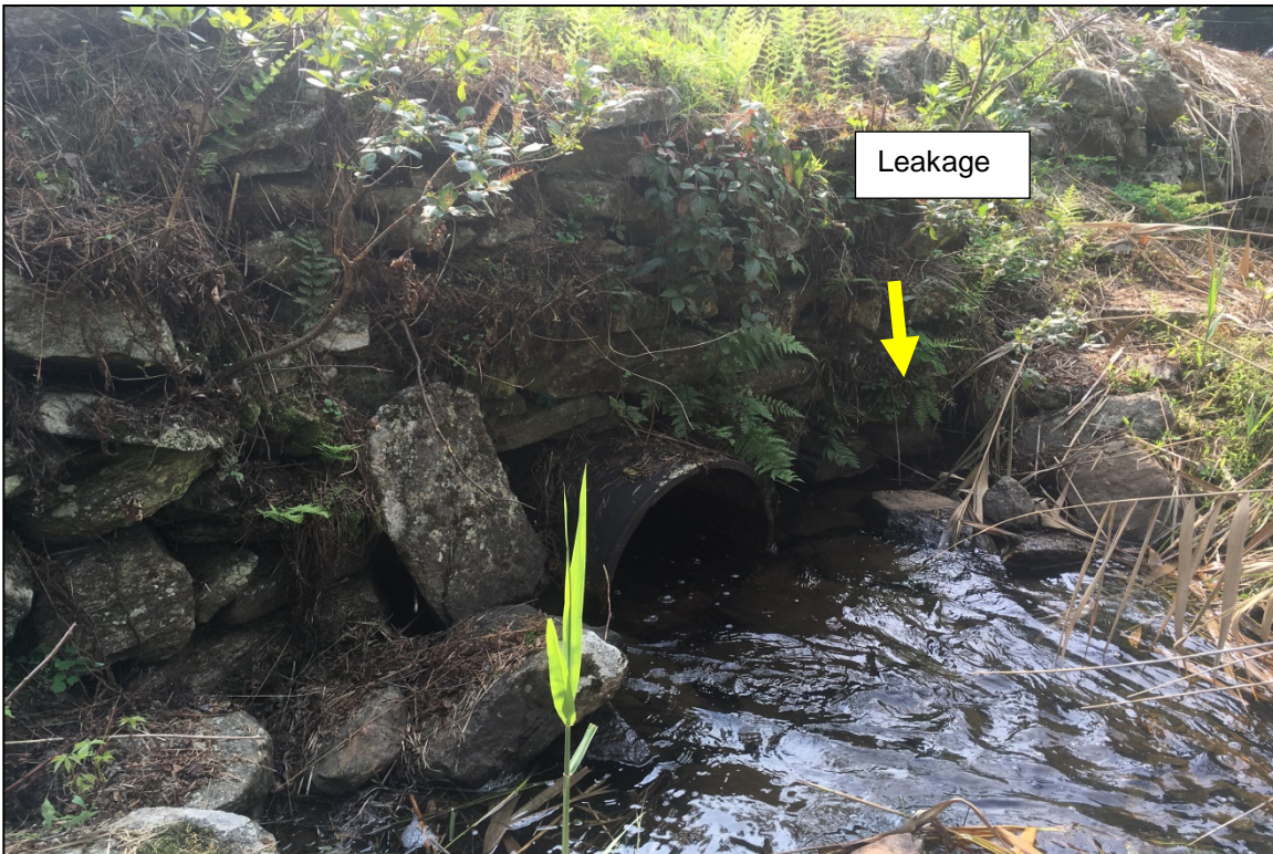
Photo 12: Overview of spillway outlet and stilling basin from downstream channel area. Leakage was subsequently observed on September 13 when the low level outlet was closed.
