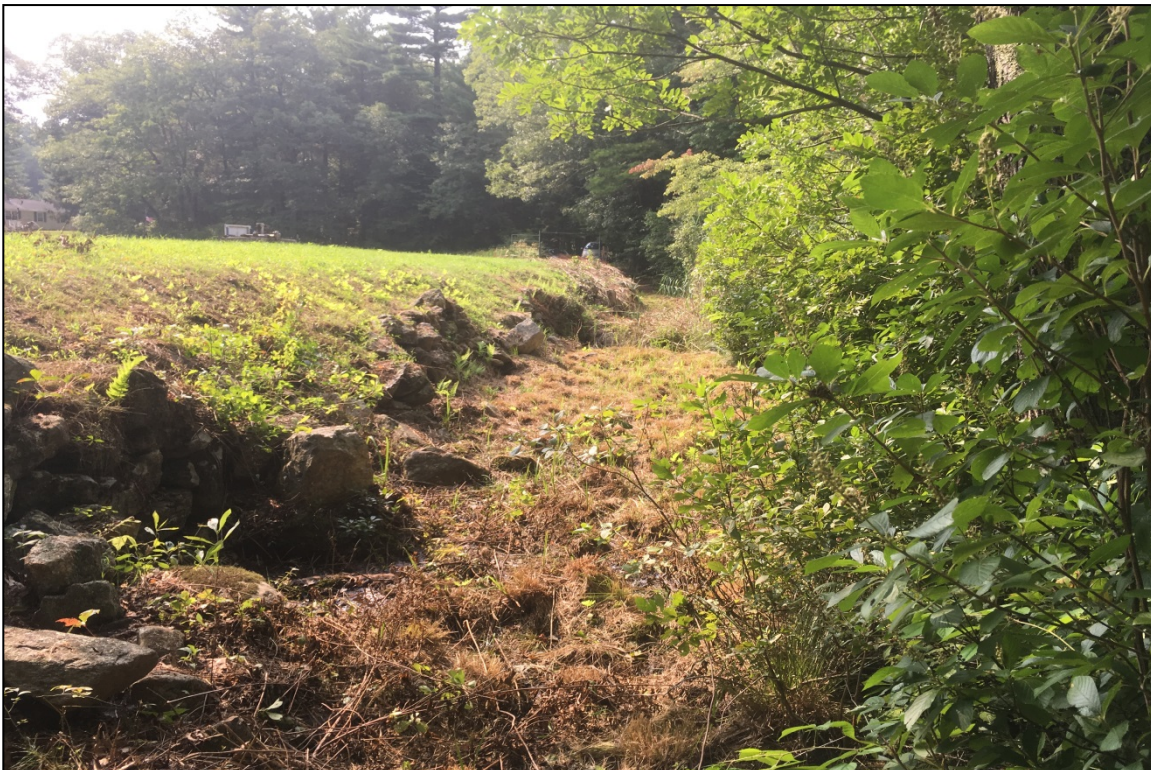
Photo 22: Areas of specific deficiencies – the downstream wall is leaning and collapsed, however, the toe is otherwise clear of vegetation.
