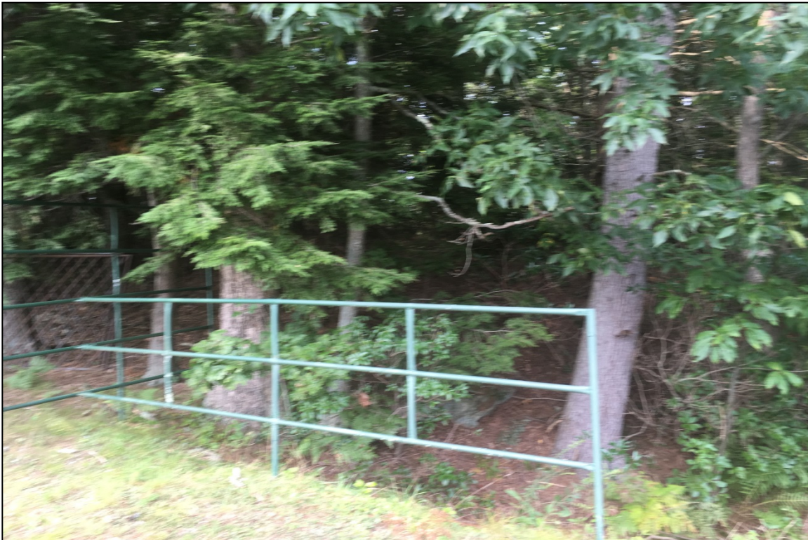
Photo 21: Areas of specific deficiencies – tree growth at the left abutment.
