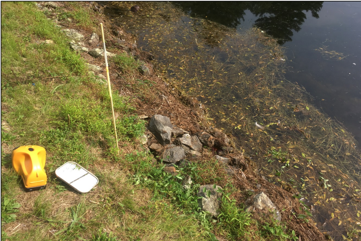
Photo 23: Areas of specific deficiencies – area of leakage entry (reported by Owner). Leakage was not detected on August 27, 2018 but was confirmed on September 13.
