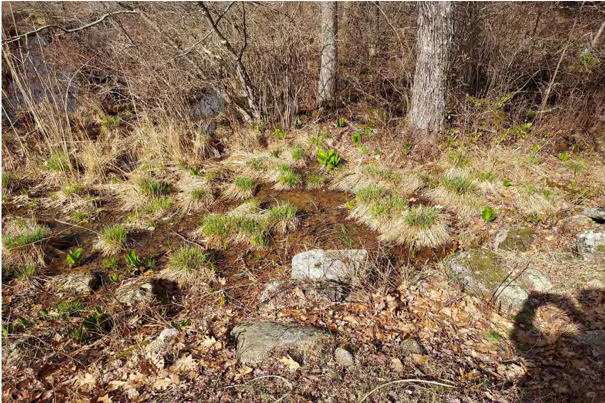
Photo 21e – A closeup of the leakage area in the previous photo, looking from the dam crest to the downstream toe area.
