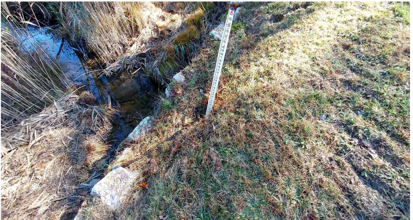
Photo 21b – A closeup of one of the holes about 2 ft. upstream of the outlet and about 1.5 ft. left of the center line of the pipe. (Photo taken 10-27-2025)
