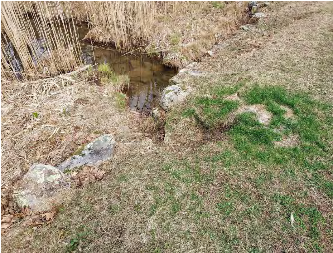
Photo 21a – Depressions and shallow holes in the vicinity of the downstream embankment area of the low level outlet pipe discharge. Note also the continued presence of a beaver slide on the left side of the outlet area. (Photo taken 04-13-2026)
