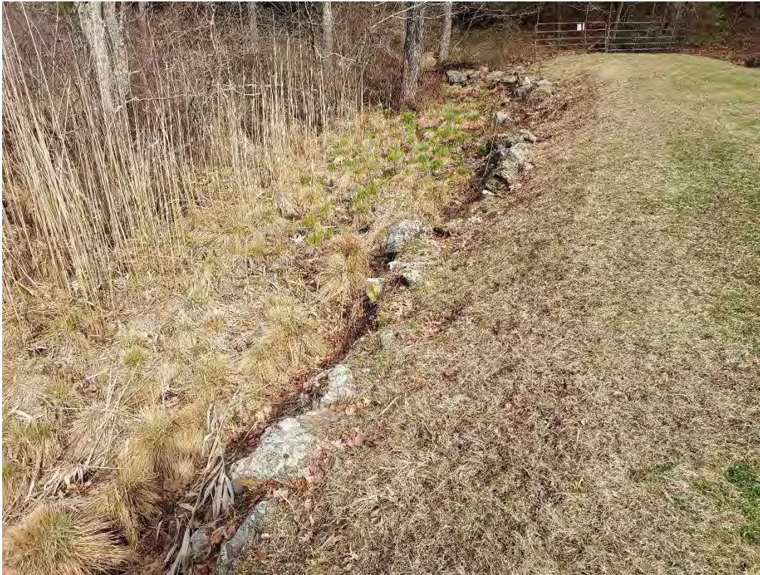
Photo 21c – A view of the downstream right side of the embankment, showing both a saturated marsh area along the base of an embankment composed of earth slope and random stone remnants from an old presumed stone retaining wall.
