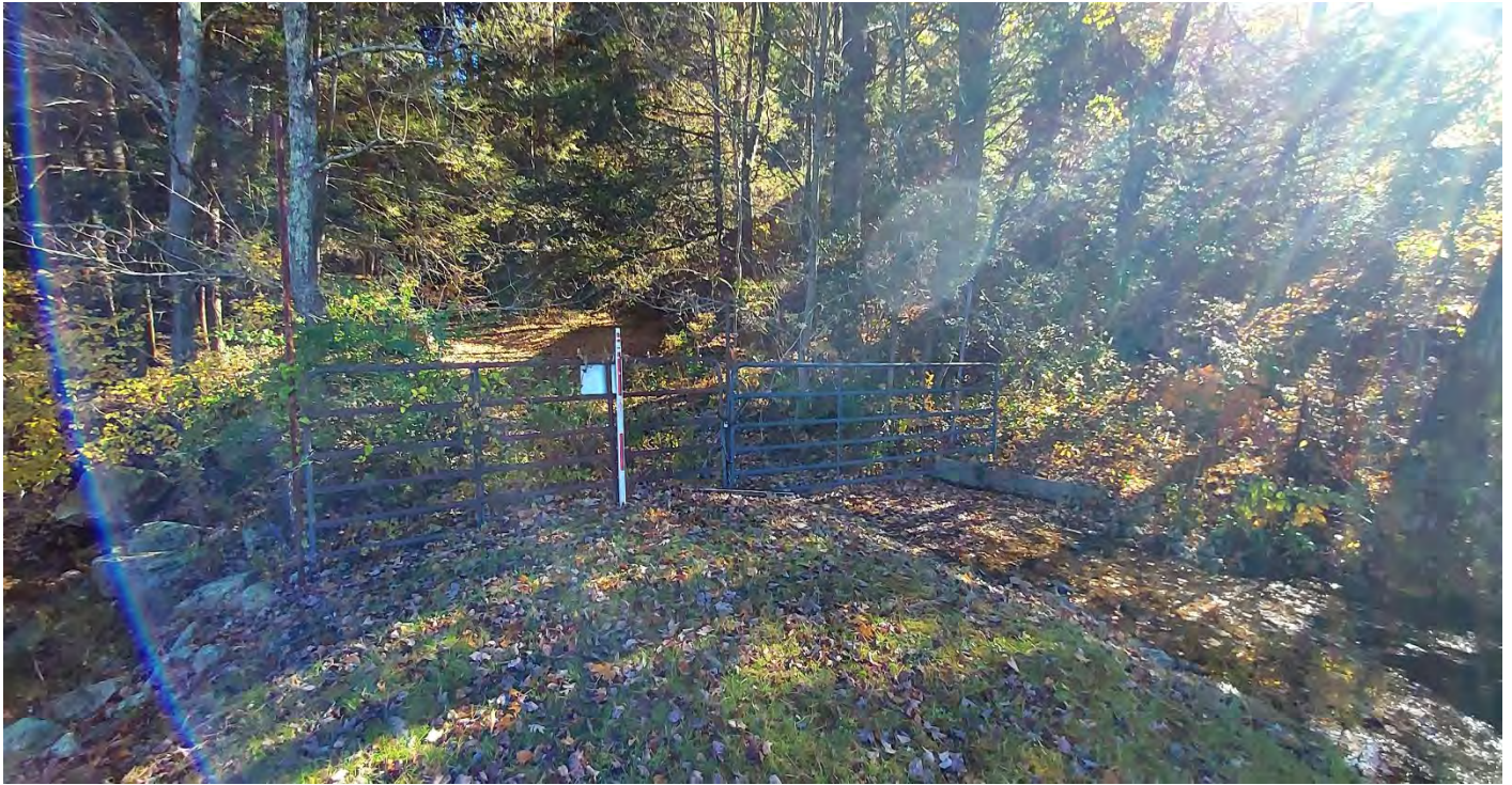
Photo 21g – Dense vegetation on the right side of the spillway, again within the 25-ft. limits of the areas to be maintained clear of trees and brush.
