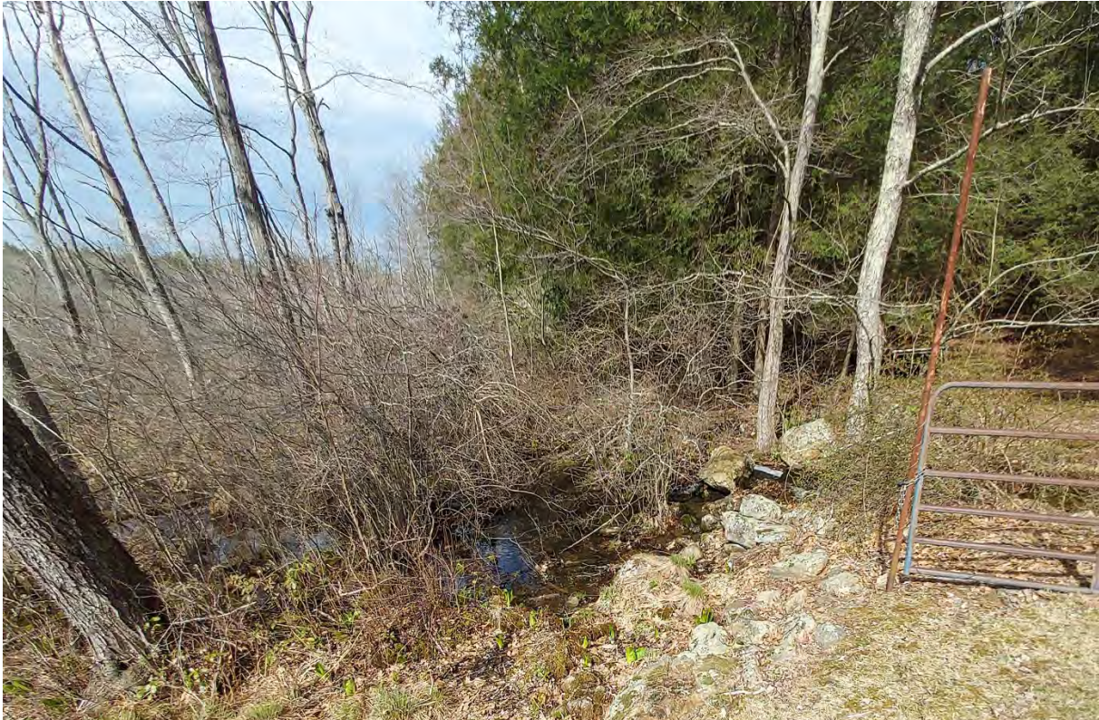
Photo 21f – Trees, brush and tall vegetation at the right downstream side of the dam and just left of the spillway discharge channel within the 25-ft. limits of the areas to be maintained clear of trees and brush.
