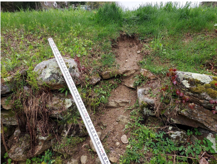
Photo 5 – Looking at the beaver slide area adjacent to the left side of the downstream pipe outlet. This area needs to be filled in and otherwise reconstructed to firm up the embankment, using on site stone and fill material from the bottom of the slide.
