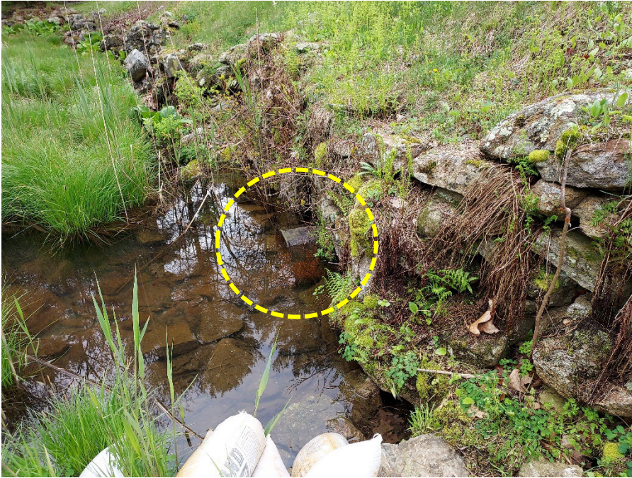
Photo 8 – The end of the low level outlet pipe at the base of the downstream stone masonry wall. Note that there were no signs of seepage from the earthen portion of the embankment and no signs of movement on the water surface at the time of inspection.
