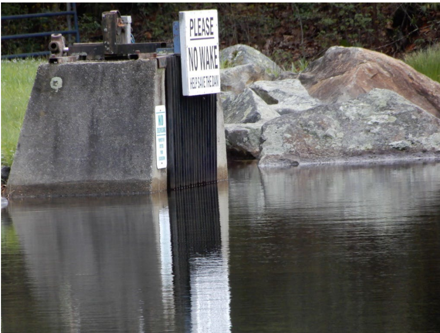
Photo 7 – The intake as seen from the upstream side, with the trash rack in place and a sign to minimize damage to the shoreline area in its vicinity.
