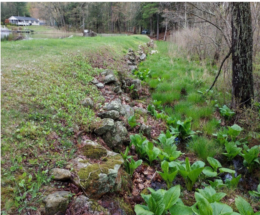
Photo 3 – The downstream side of the embankment as seen looking from the right to the left side. Note the extension of the grass area to approximately halfway down the slope along most of the length of the dam.
