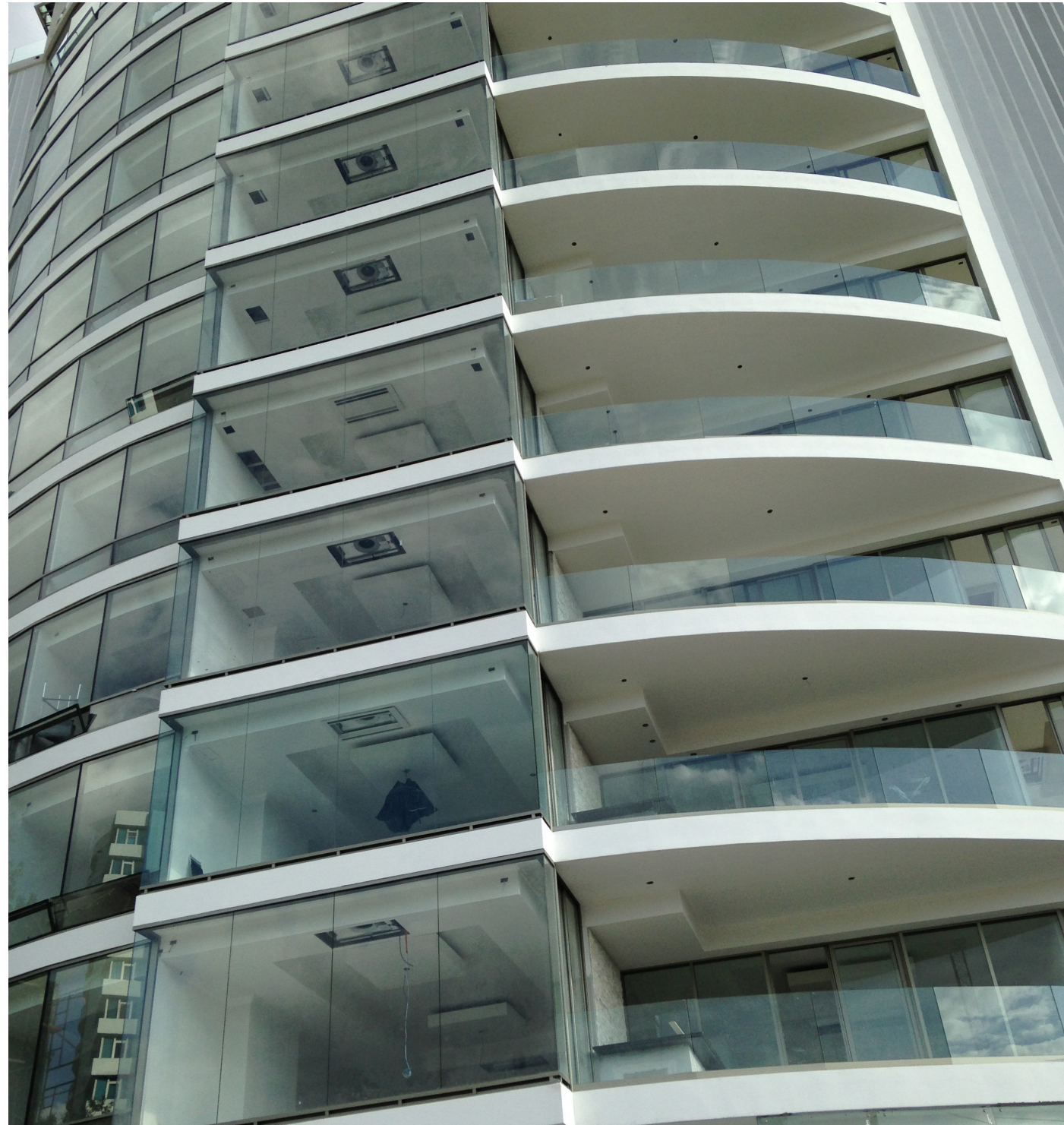
Main facade, vertical element design and construction method was designed by myself on site.
