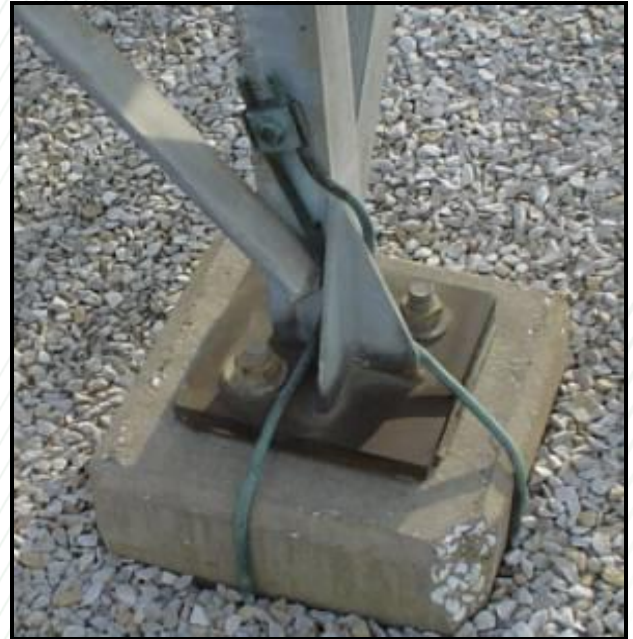
Tower Properly Grounded
