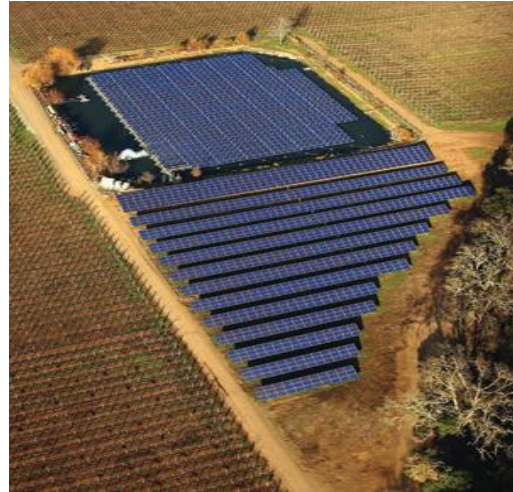
Figure 8: A 477kWp mixed ground-mounted, water mounted system in Napa County, California.
