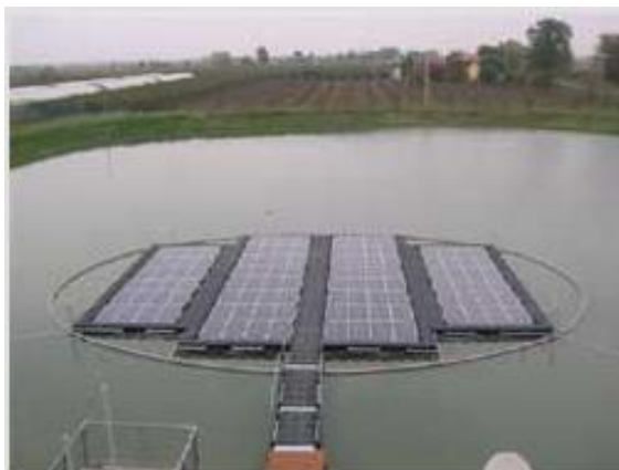
Figure 7: System at Solaralo, Italy. (From: http://www.luceonline.it/web/en/ricerca/costruzione-del-primo-impianto-fotovoltaico-galleggiante-in-puglia/ )
