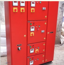
Control Panel for Fire Pump
