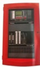
Addressable Fire Alarm Panel
