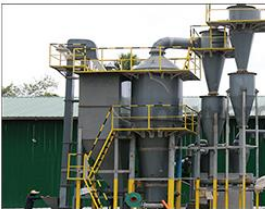
0.5MW CFBG POWER PLANT-2
