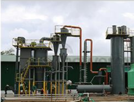
0.5MW CFBG POWER PLANT
