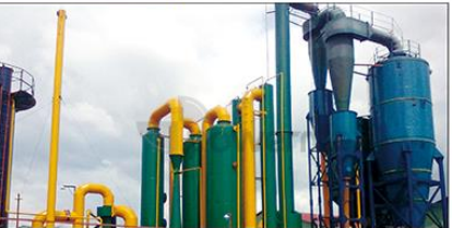
1.5MW CFBG POWER PLANT
