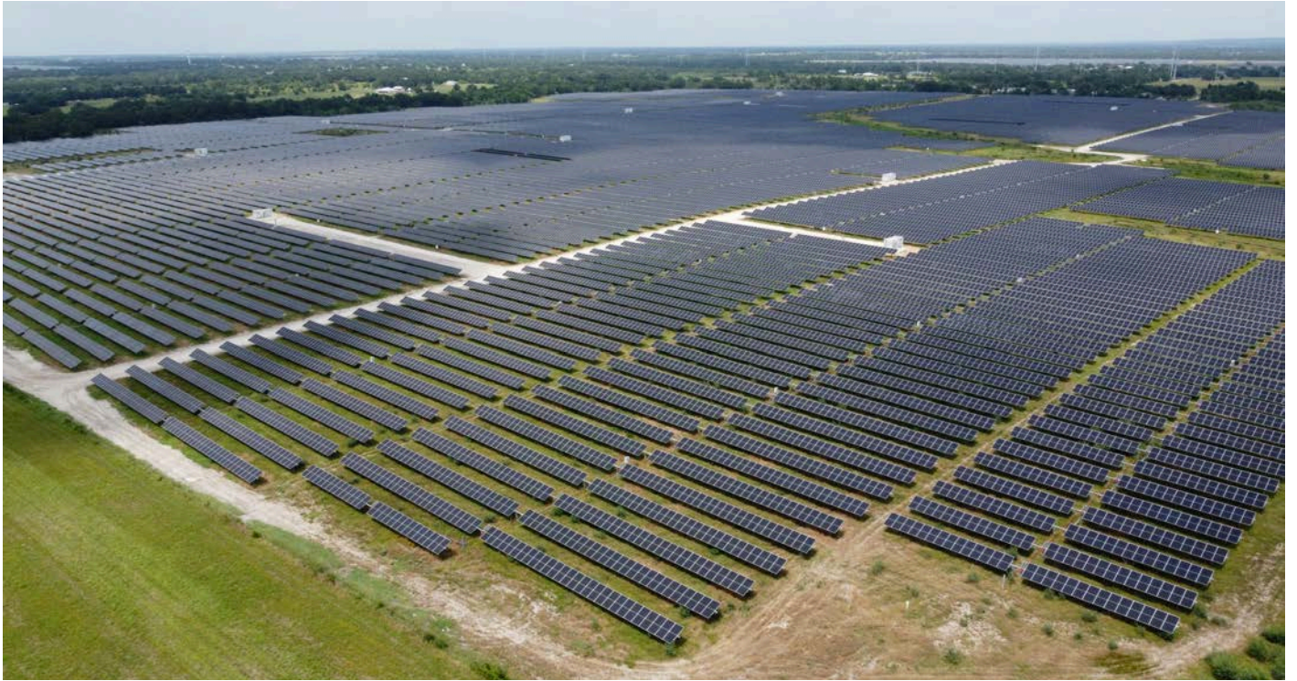
Grimes Solar Project (210 MW)
