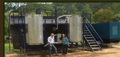
2021 - extraction plant, commissioned/ready
