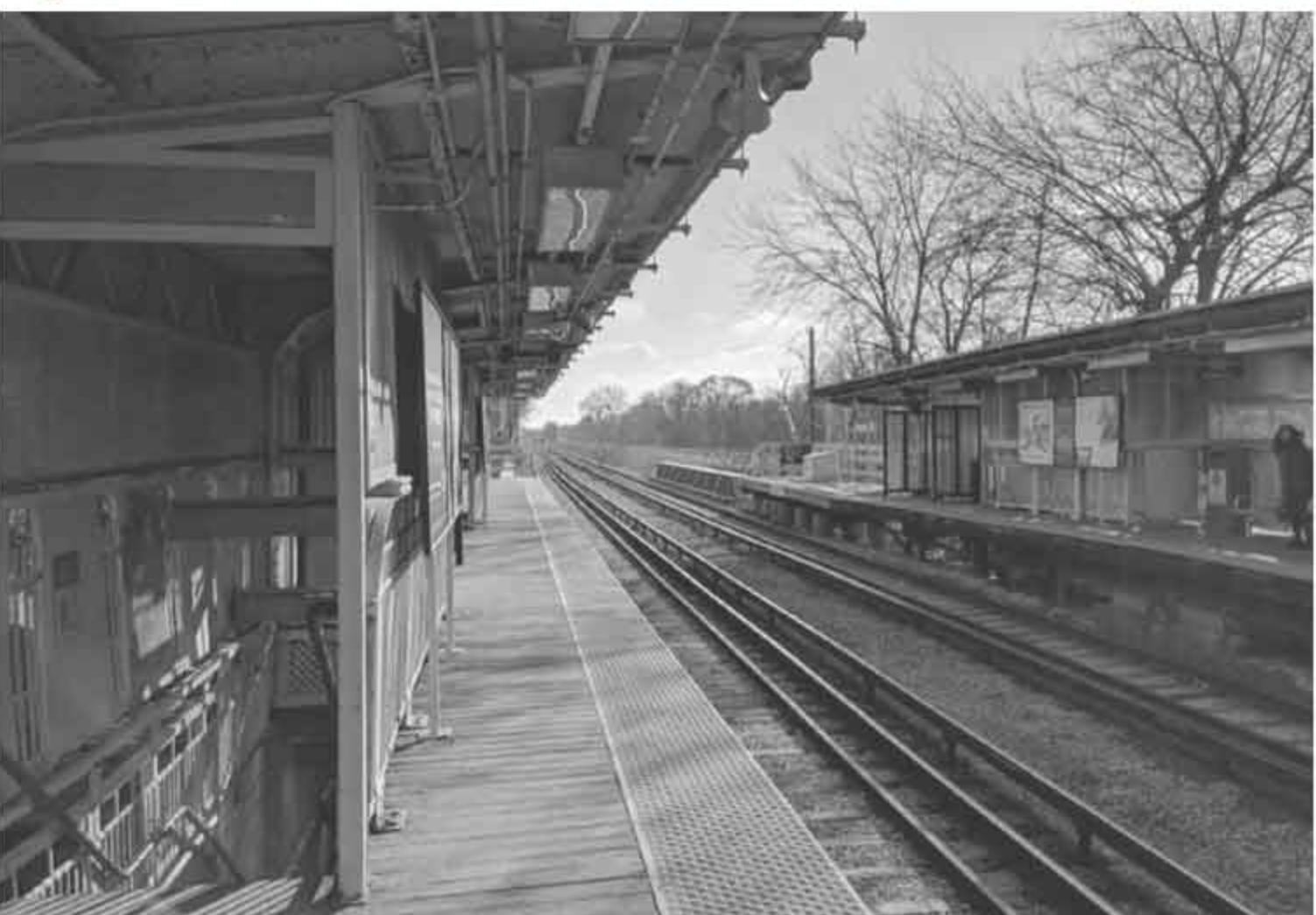
Non-accessible elevated train platform in the winter, 2025.
