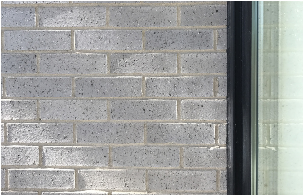
Image 37: Brick Cuts on Inside Corner.
