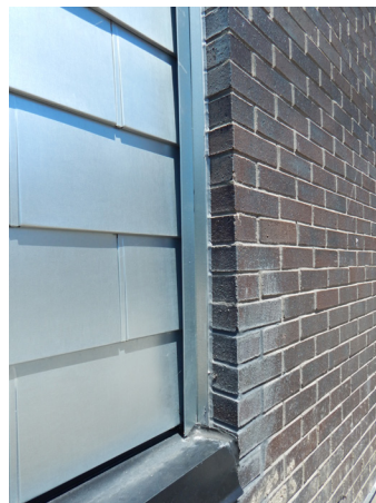
Image 56: 1620 Central Brick Condition at Window.
