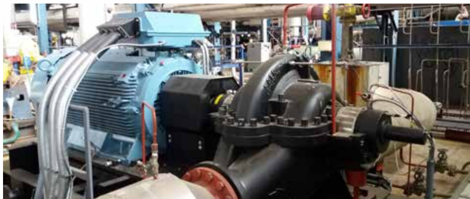
NR. 2 SKDZ-4P 250-750 1000kW SERBIA DISTRICT HEATING
