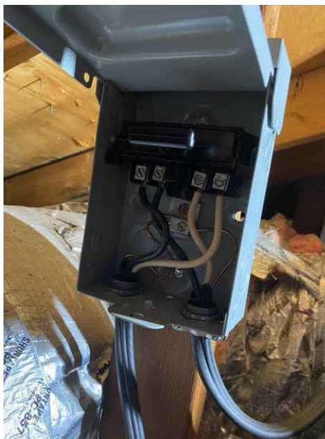
Disconnect for air handler
