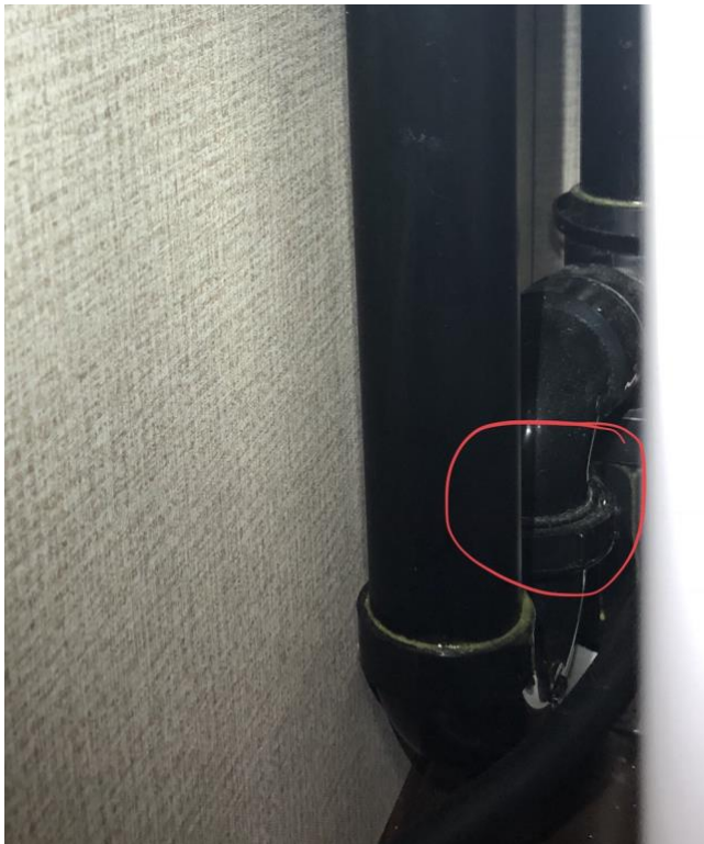
Figure 1: Water was leaking from this fitting.
