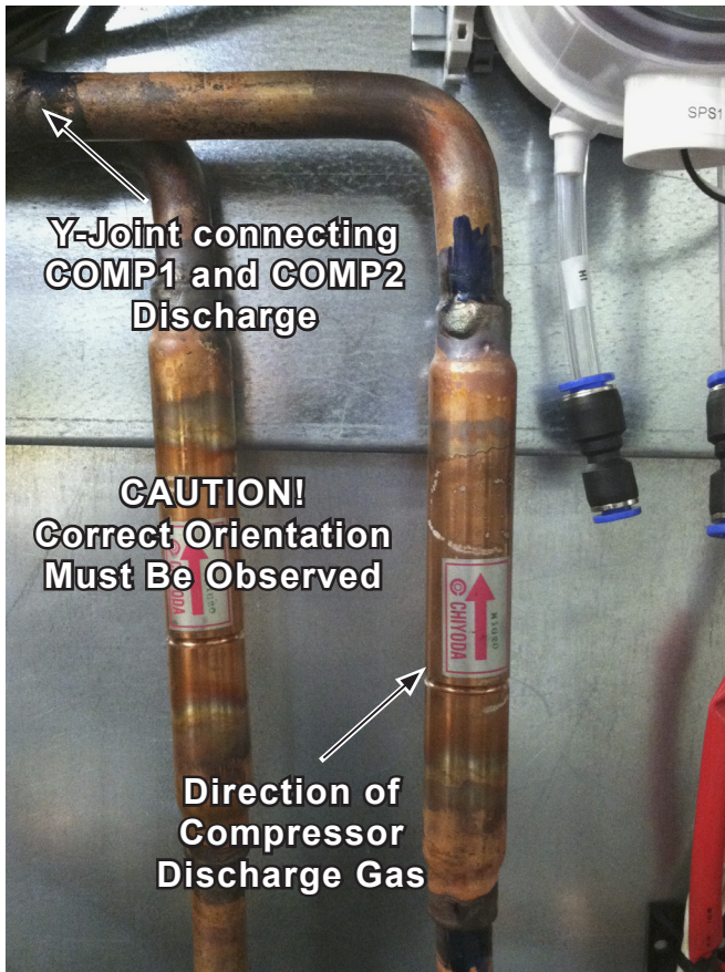
Figure 26: Discharge Line Check Valves on Large Cabinet (7.5T) Heat Pump (DPH)
