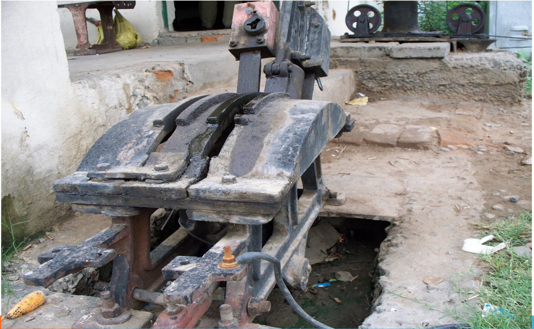
EARTHING OF LEVEL CROSSING GATE LEVER FARIDABAD – NORTHERN RAILWAY YEAR 2007
