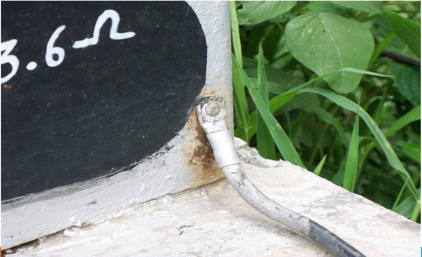
EARTHING OF LOCATION BOX GHAZIABAD – NORTHERN RAILWAY YEAR 2006
