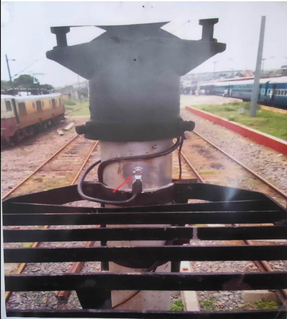
Earth Bond Installed on Signal Mast at Sonpur Railway Station on 12 July 2017
