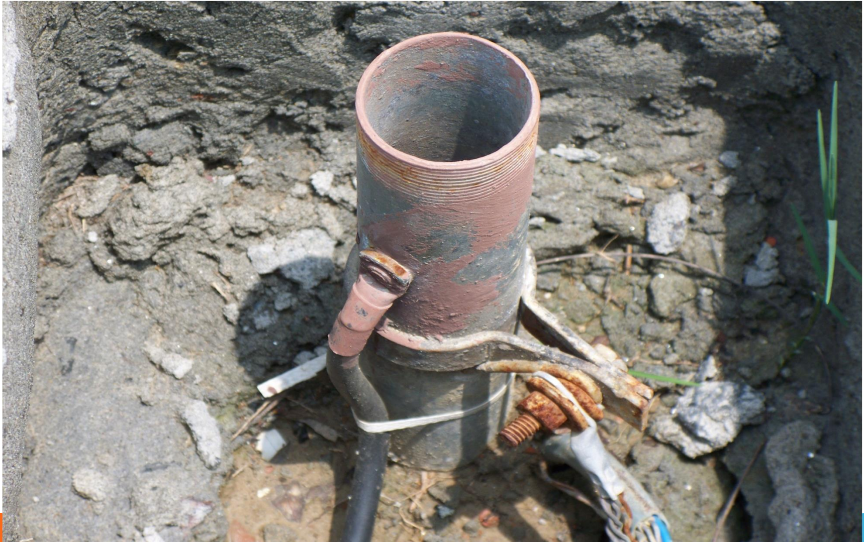
PINBRAZED CONNECTION ON EARTH ELECTRODE - G.I.PIPE ROHTAK – NORTHERN RAILWAY - YEAR 2007
