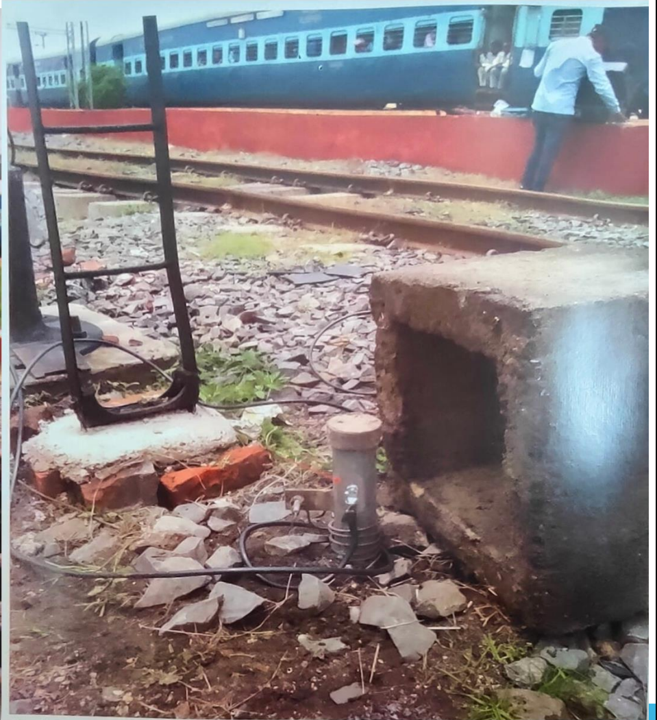
Earth Bond Installed on GI earth at Sonpur Railway Station on 12 July 2017 by Pin Brazing
