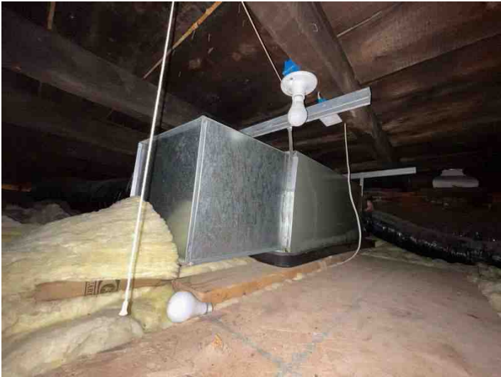
Utility - Heater In Attic
