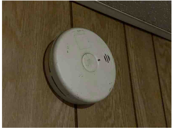
Smoke and Carbon Monoxide Detector
