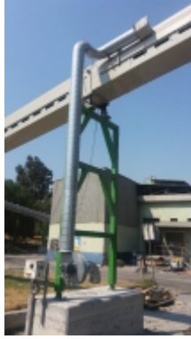
Blower arrangement for belt lifting
