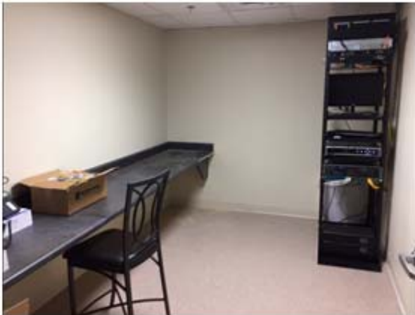
VIEW OF TYPICAL IT/SUPPORT ROOM
