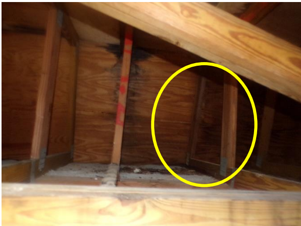
View of water staining on roof sheathing.
