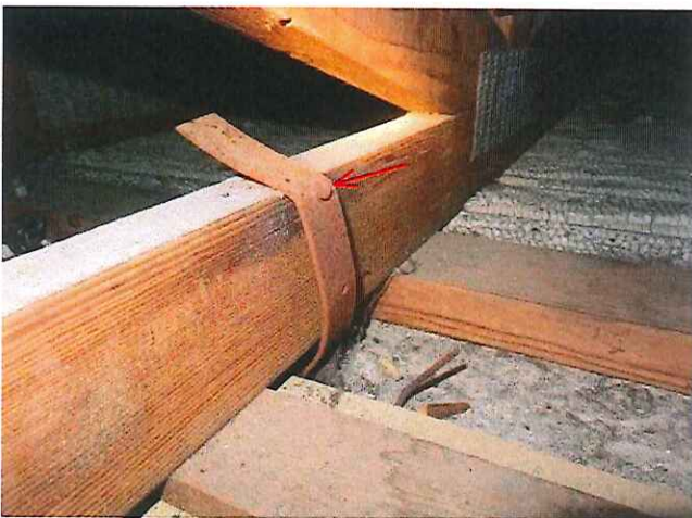
#5 Clips for roof to wall attachment with less than three nails
