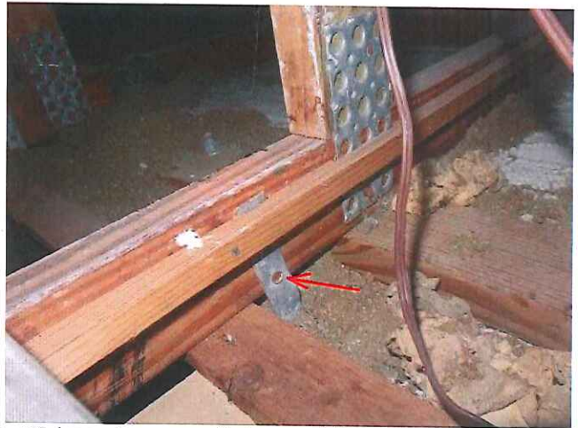
#8 Clips for roof to wall attachment with less than three nails
