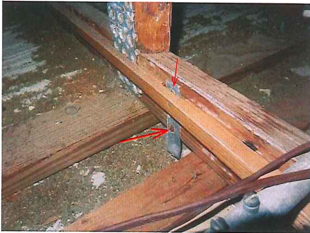
#7 Clips for roof to wall attachment with less than three nails
