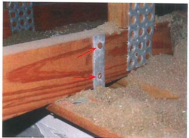
#6 Clips for roof to wall attachment with less than three nails
