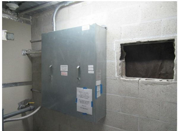
View of missing section of CMU wall.
