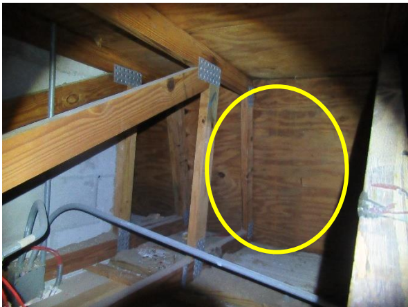
View of water staining on roof sheathing.
