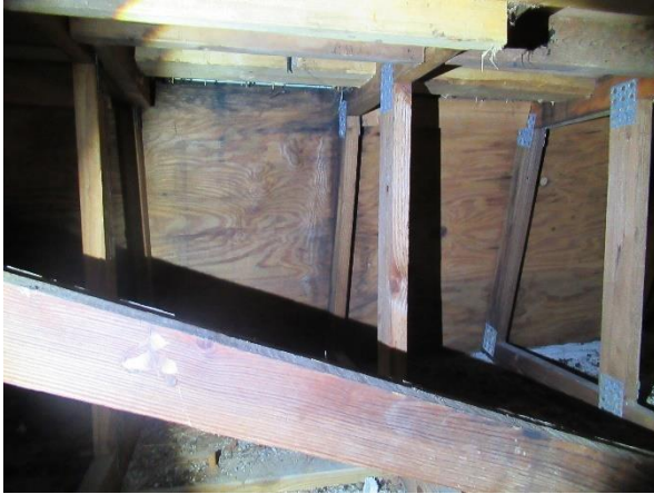
Partial view of attic and water staining on sheathing.
