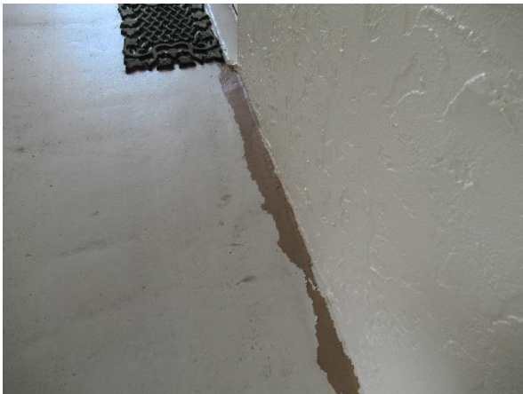
Typical breezeway chipped coating.
