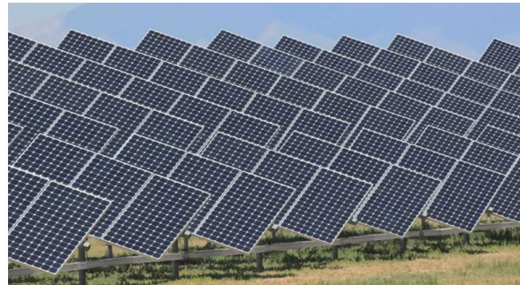
Xcel Energy's Sandhill Solar Farm, CO.
