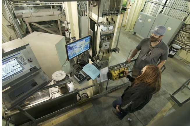
Integrated Waste Treatment Unit (IWTU) operator Samantha Phillips maneuvers a crane at the facility at DOE's Idaho Cleanup Project while Trevor Clark, another IWTU operator, observes.
