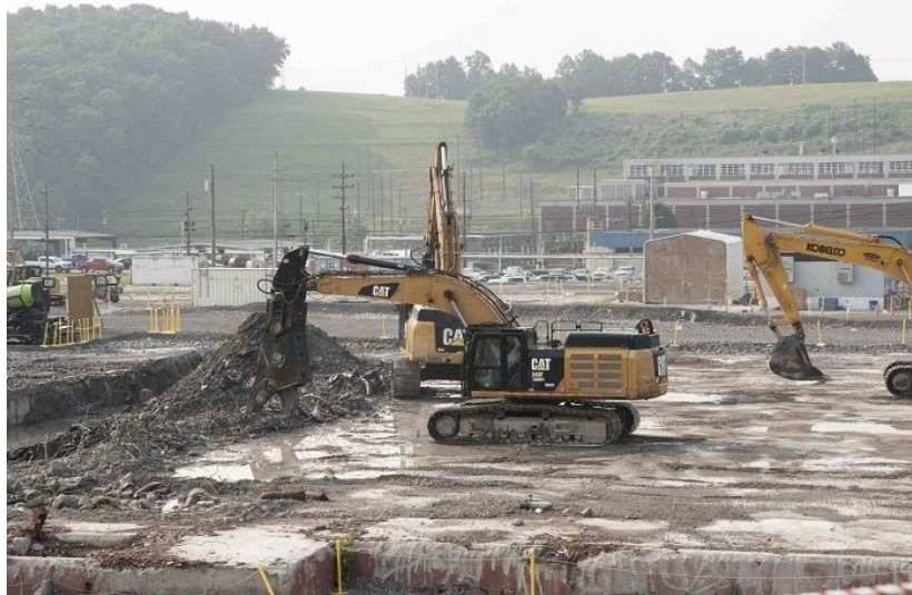
Workers are in the final stages of removing the Biology Complex slab at the Y-12 National Security Complex. This makes available the complex's 18-acre footprint for use by the NNSA to support national security missions.
