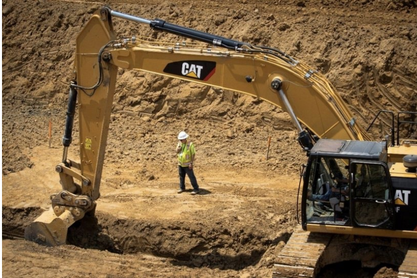
The first excavation of soil got underway in summer 2021 to remove sources of potential groundwater contamination and provide fill dirt for the On-Site Waste Disposal Facility at the Portsmouth Site.
