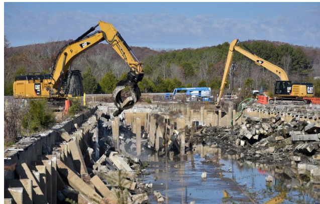
Crews removed concrete subsurface structures of the K-832 basin at Oak Ridge in 2019 and pumped nearly 2 million gallons of water from the basin before beginning demolitions.
