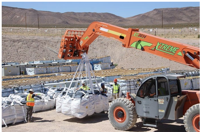
Crews placing containers of waste into the Radioactive Waste Management Complex at NNSA.
